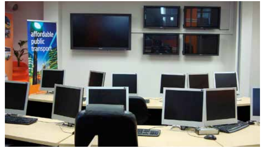
Computer equipment supplied by the consultant remains unused at the IFM and ITS systems' control room (view from the back)
